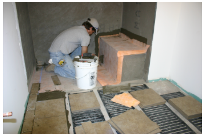
Heating on the floor and the bench
