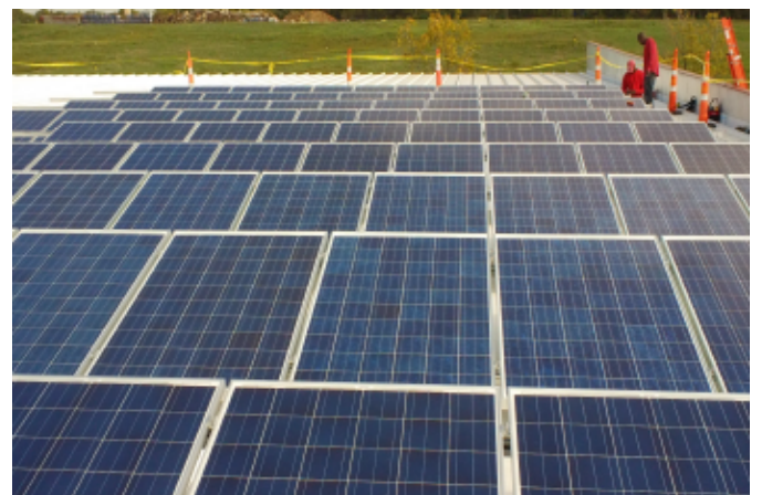
Solar Panles on Roof
